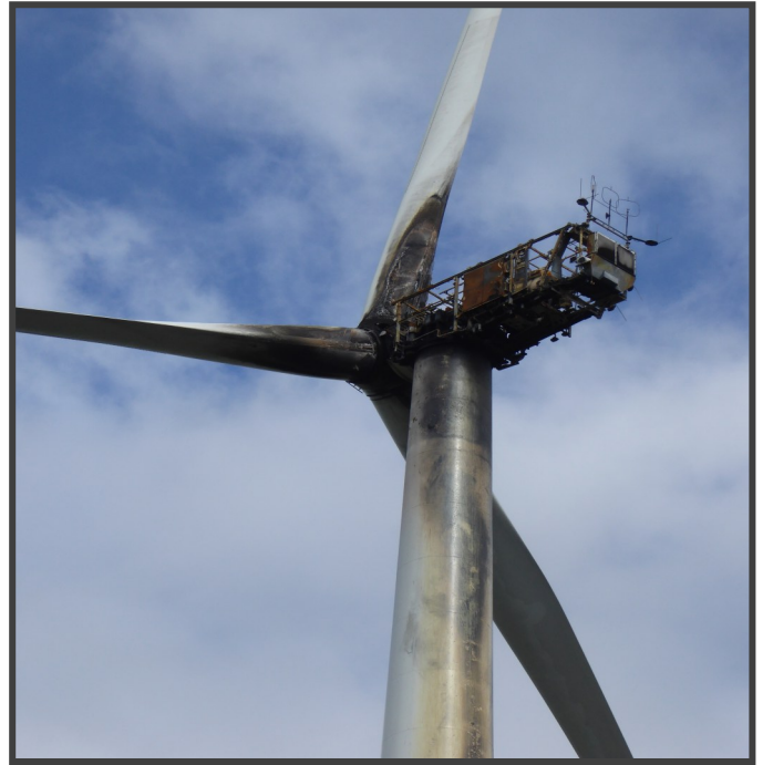
Wind Turbine Failure, U.K.
