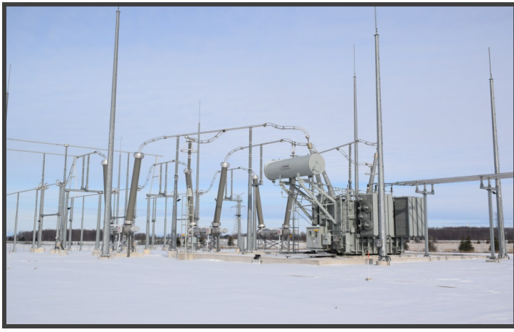
Wind Farm HV Substation, Canada
